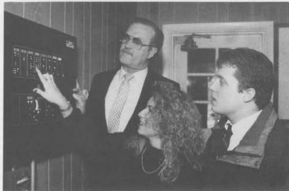
Wayne Carlile (left), Director of Safety and Security, demonstrates a fire alarm system at Angelus Hall to resident assistants Anne Gendron '92 and Craig Austin '92.
