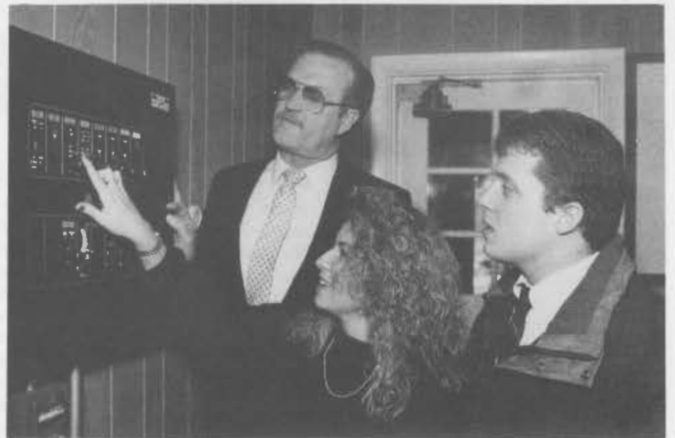
Wayne Carlile (left), Director of Safety and Security, demonstrates a fire alarm system at Angelus Hall to resident assistants Anne Gendron '92 and Craig Austin '92.
